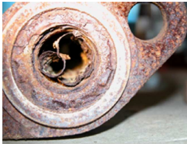
Fig. 2. Corrosion buildup in chlorine repackaging piping system.
